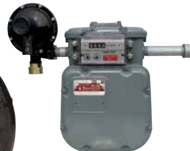
Attached to Vapor Meter
